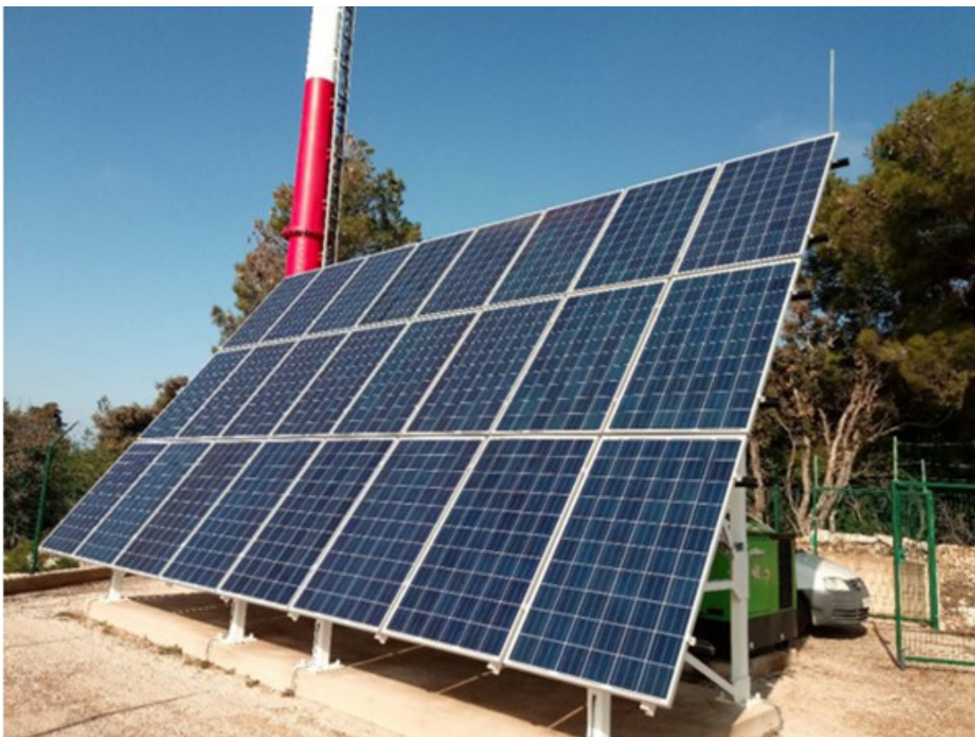
Figure 5: Ground-based navigation facility (DME - Distance Measuring Equipment) on Lošinj Island, Croatia, powered primarily by solar energy (Photo courtesy of Croatia Control).
